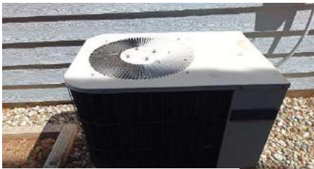
Exterior heat exchanger / AC Equipment is original and should be monitored due to age. Equipment was tested with thermal imaging.
