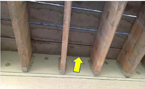
No deck to wall flashings noted
