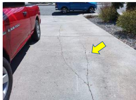
Example: Driveway shows degree's of cracking. Monitor*
