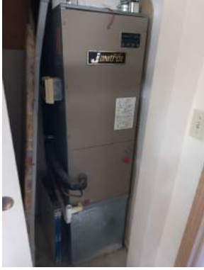
Furnace Equipment was tested with thermal imaging.
