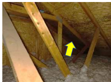
Example: Areas of minor mildew, moisture impact noted to sheeting . Monitor*
