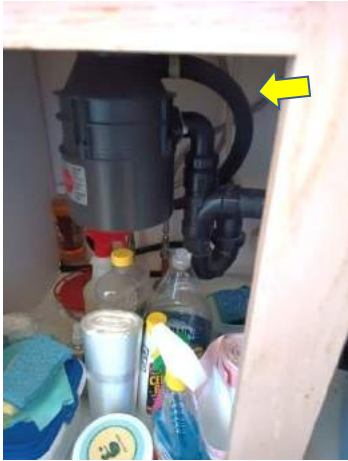
Improper routing of dishwasher drain line. Education /update to high loop is recommended
