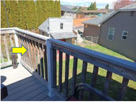
Finish at deck railings show heavy wear.
