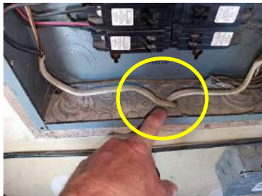
No compression collar / insulator on wire entering panel.
