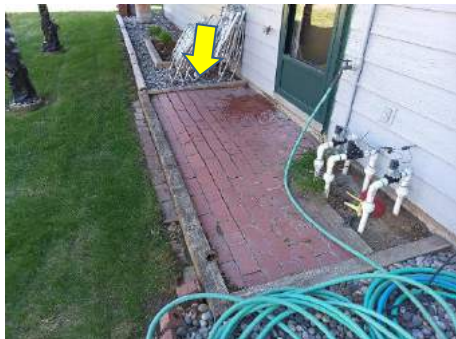
Brick paver patio shows degree's of settling Monitor
