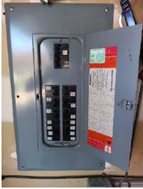
Service Panel at Garage
