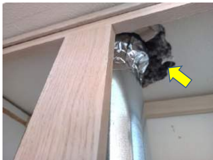
Seal oversized penetration for vent pipe at cabinet over range.
